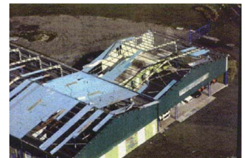
Loss of corrugated, metal, roof sheets
