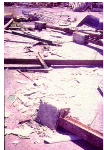
Foundation (too small for light weight building) pulled completely out of ground
