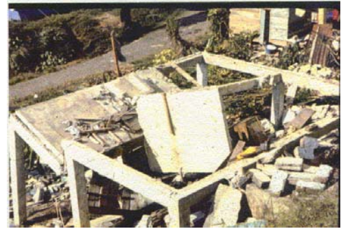
Total loss of unreinforced concrete block walls and destruction of reinforced concrete supports
