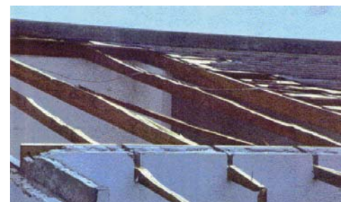
Longitudinal splitting of timber rafters
